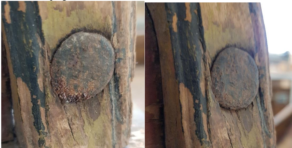
(A rivet before and after mechanical removal of the weeping corrosion)
